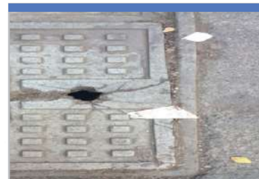
Condition of the Regular keyhole lifting arrangement of other make FRP manhole covers
